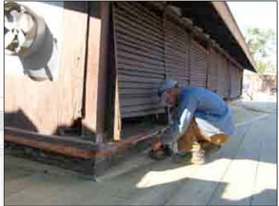
Nathan Harris installs a cricket on the north side of the monitor.
