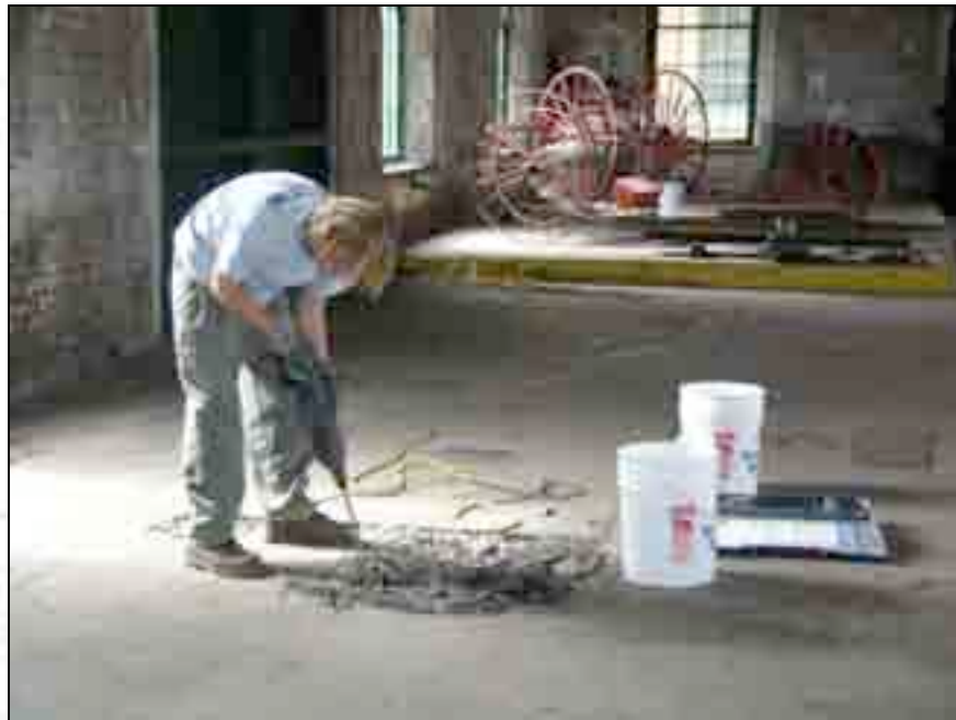
Historic Masonry Specialist Travis Brown drills away deteriorated concrete in order to repair it.
