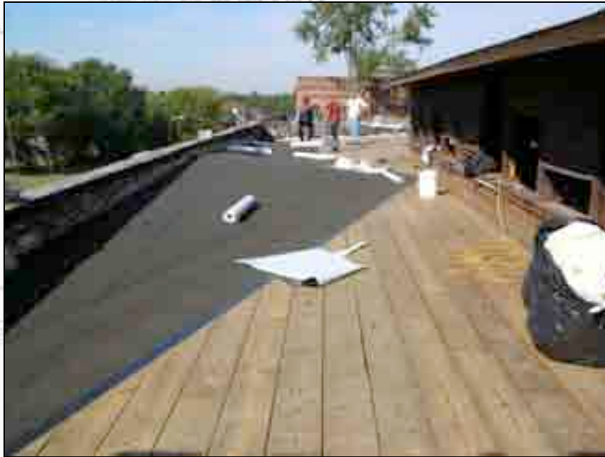
A roofing membrane was installed with the assistance of John Herdina, roofing consultant.
