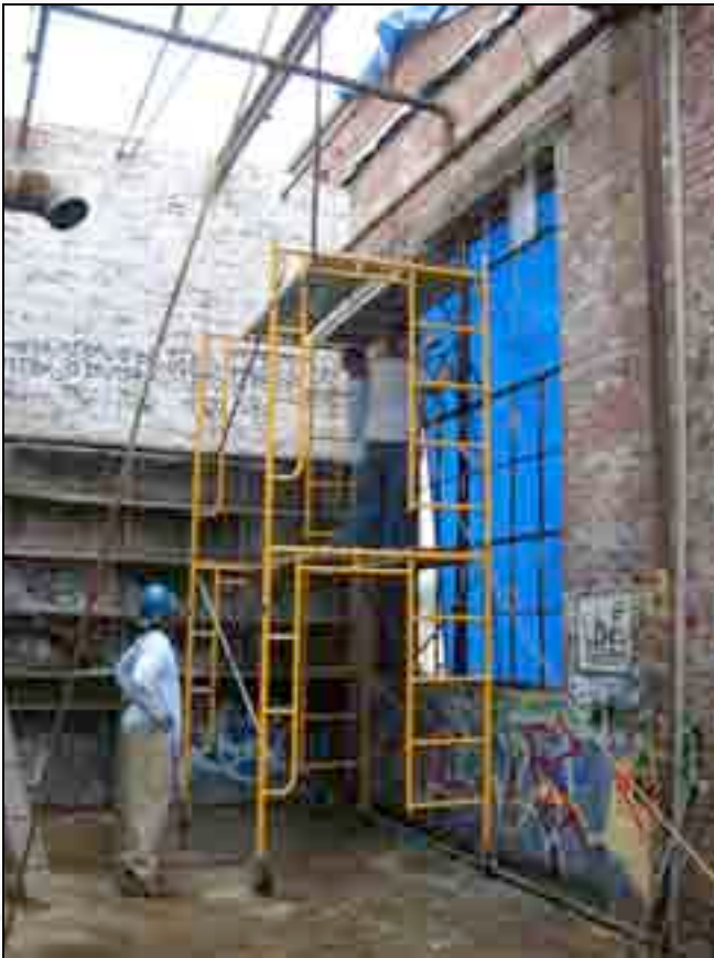
Chris Latson, Joe Rothwell, and Tim Gaffney remove a window from the interior west wall of the Paint Shop.
