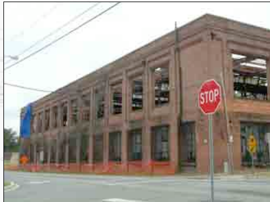
Current view of west façade with most of the main floor windows removed.
