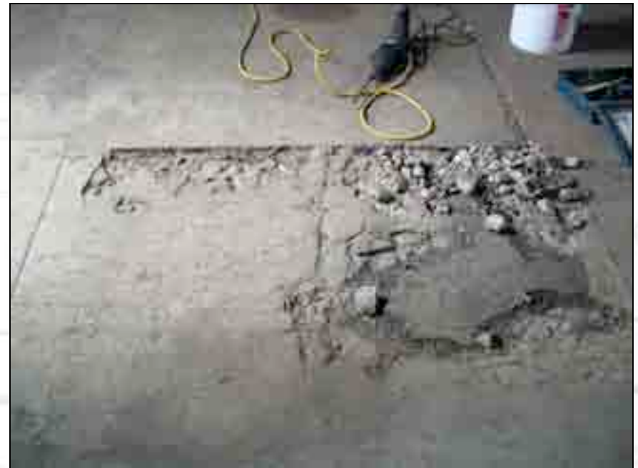
Close-up view of deteriorated concrete.
