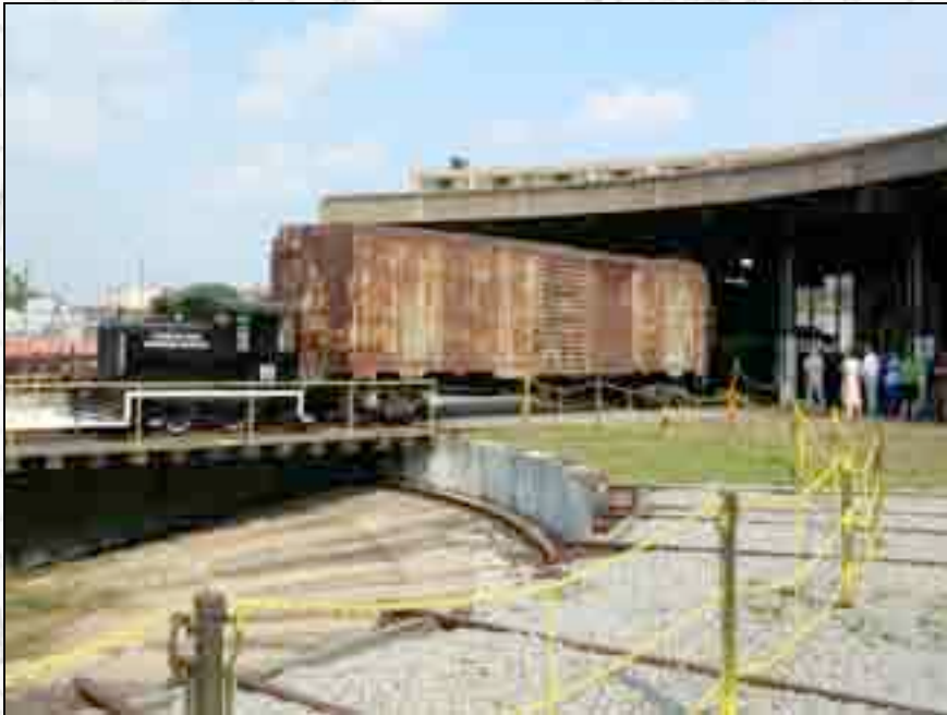
Terry Koller shoves an historic boxcar into the lane with the nearly completed pit cover.
