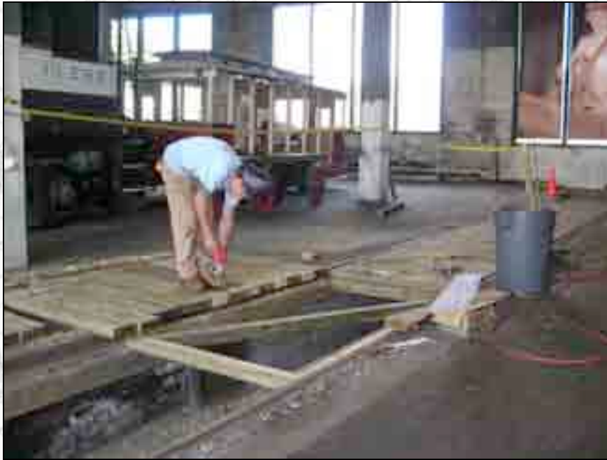
Preservation Team member Joe Lyons helps construct a pit cover for one of the lanes.
