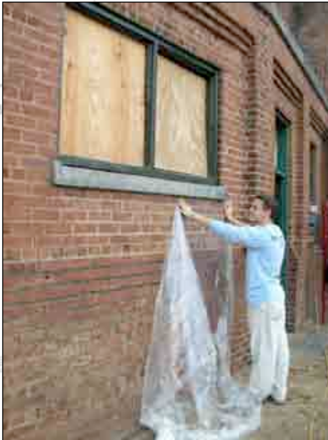
Jason Cobb applies a plastic covering to protect the building from paint remover.
