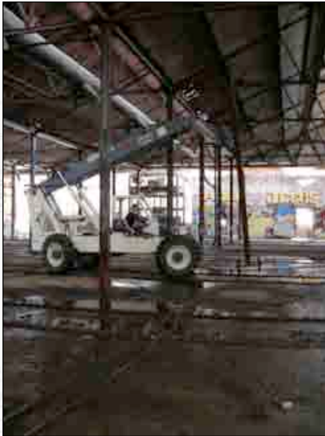
Brady Warner moves a repaired steel column back to its original placement.
