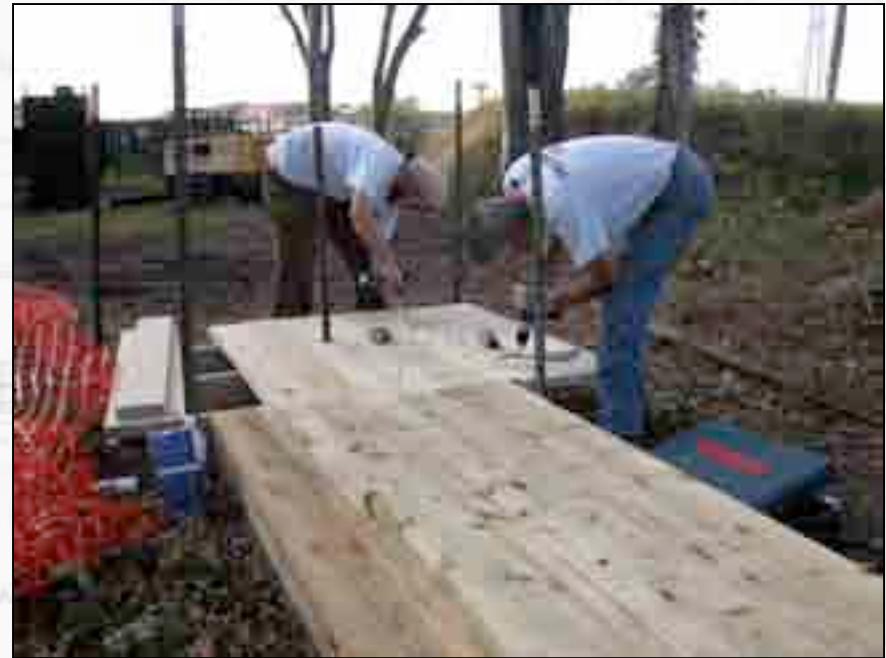
View of east manhole. Nathan Harris and Charles Adkins secure a cover over the t-shaped manhole.
