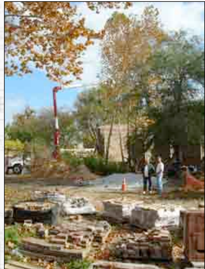
North view of area during tree removal. The Carpentry Shop can be seen on the right.
