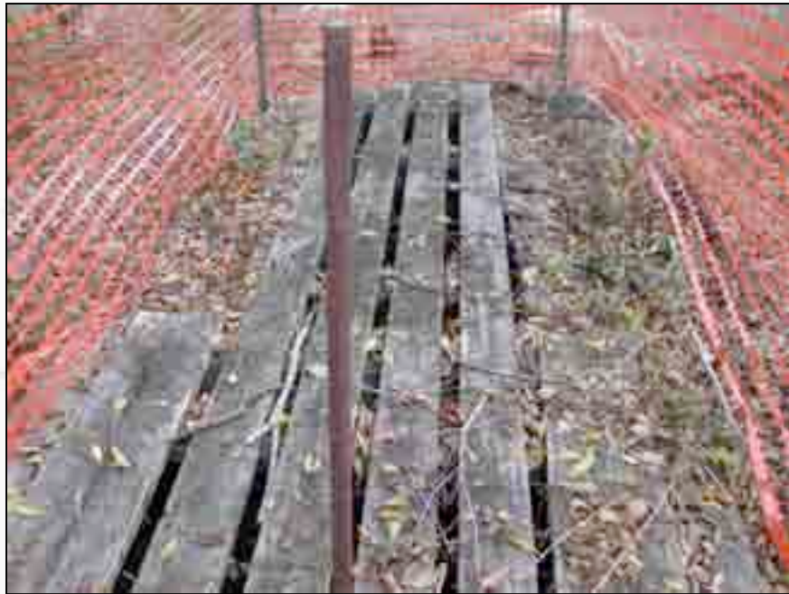
Severely deteriorated t-shaped manhole cover located at the east of the Paint Shop.
