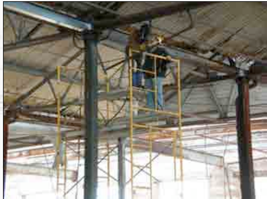
Preservation Team members weld structural steel elements at the sawtooth roof area.
