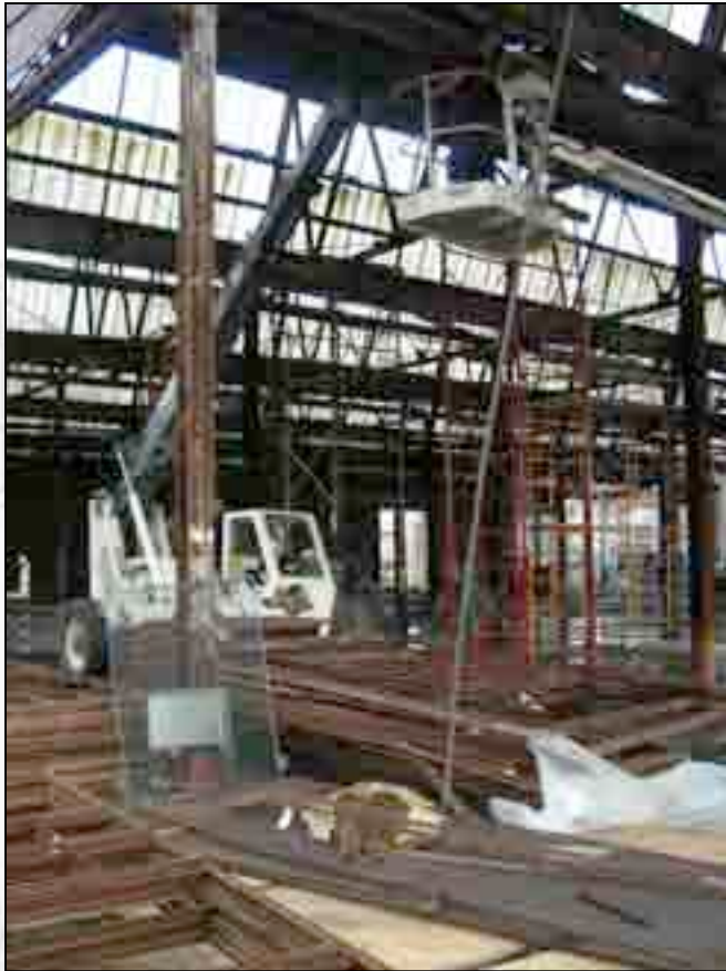
Justin Rowles installs the last replacement beam as Brady Warner assists with the forklift.
