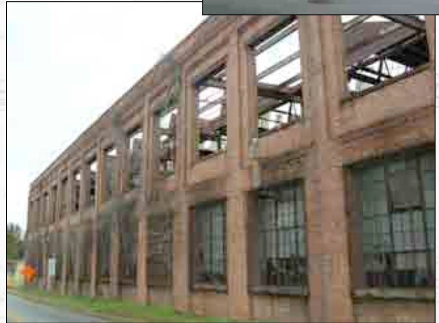
Current view. All of the windows from the main floor have been removed. Interpretive panels will be installed in some of the openings.
