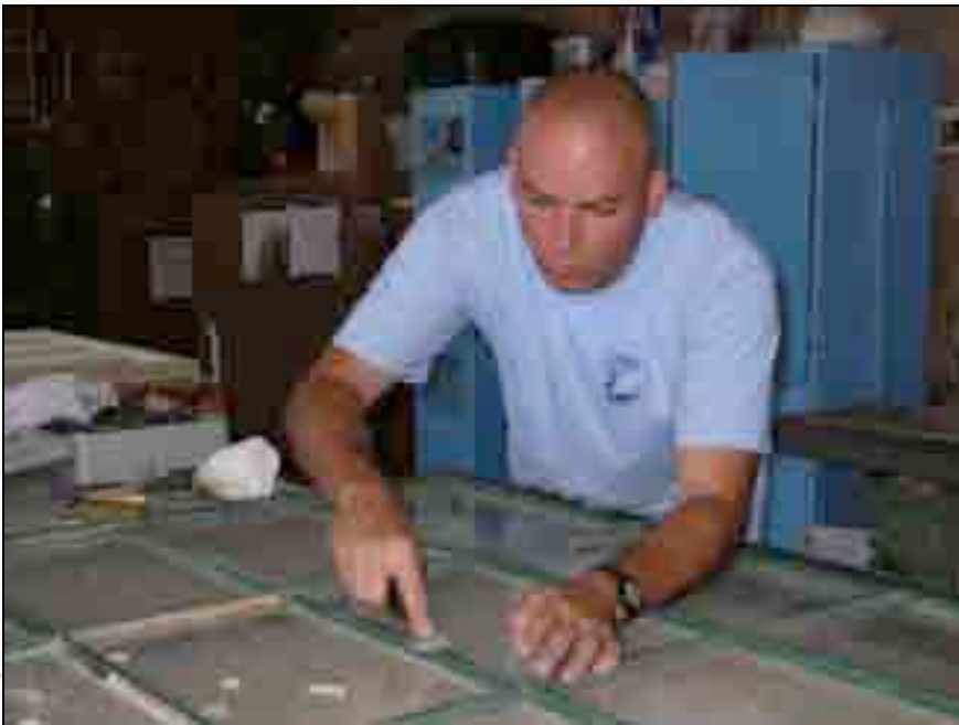
Kurt removes the deteriorated glazing on a window from the first floor of the Tender Frame Shop.
