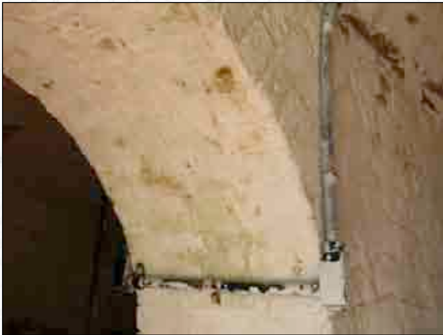
Before mold was removed
