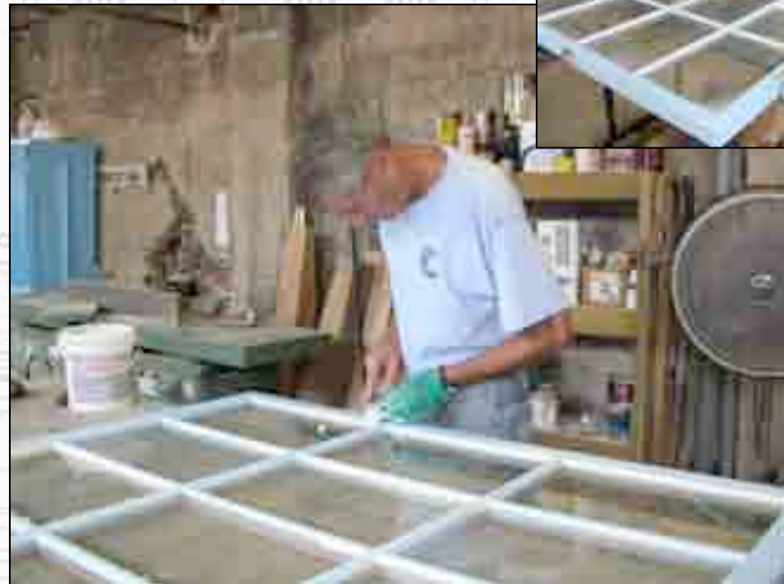
After the deteriorated glazing is removed, new glazing is applied. Charles is shown reglazing a window.
