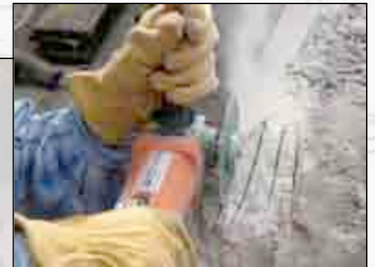
Amy Grace cuts hatch marks into the concrete sill in order to remove areas of rust jacking.
