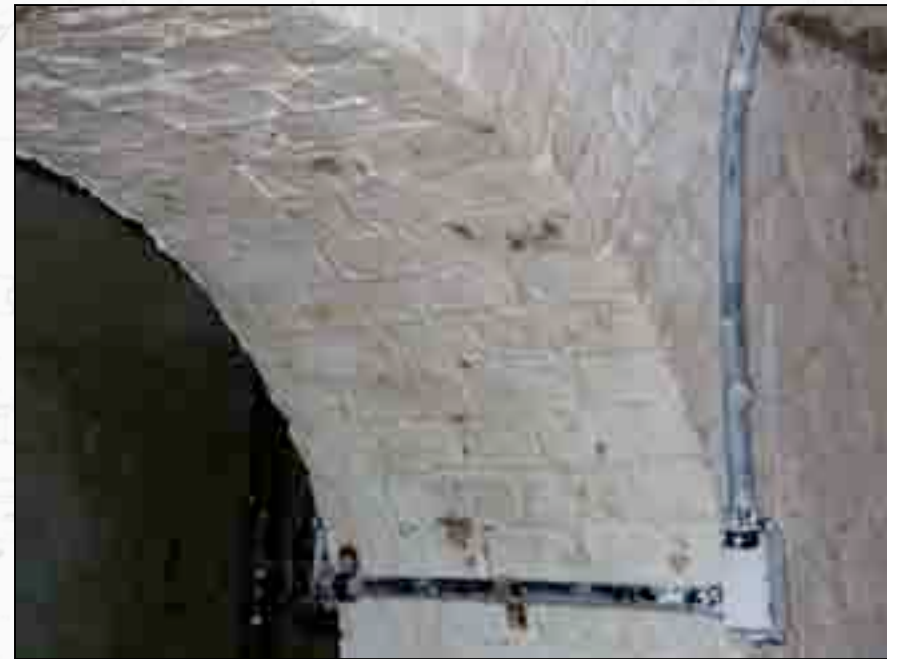
After it was cleaned
