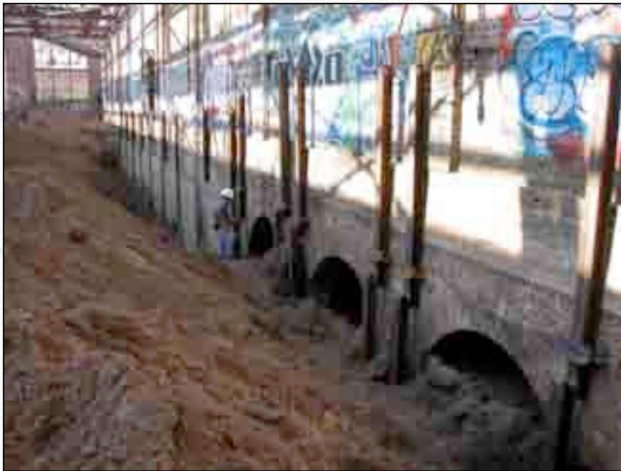
CHS and Winter Construction work together to install barriers to retain soil between the Coach Shop and Paint Shop Basement.
