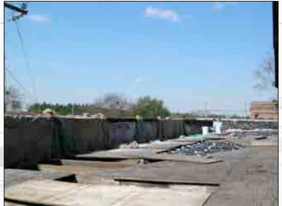
Repointing is being done on the west end of the parapet wall.
