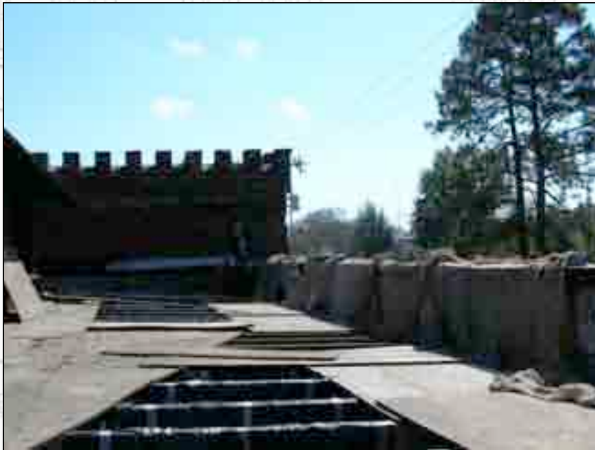
Areas along the parapet wall have been repointed and are now covered with burlap.
