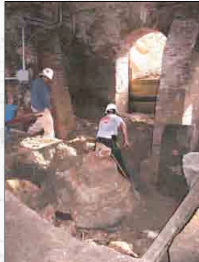
Winter Construction completes soil removal along east wall of Paint Shop basement.
