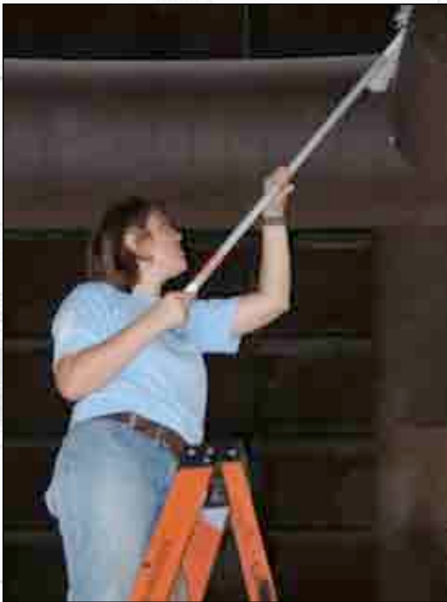
Lissa cleans the exterior surfaces of the air ducts in the ceiling space above the office.
