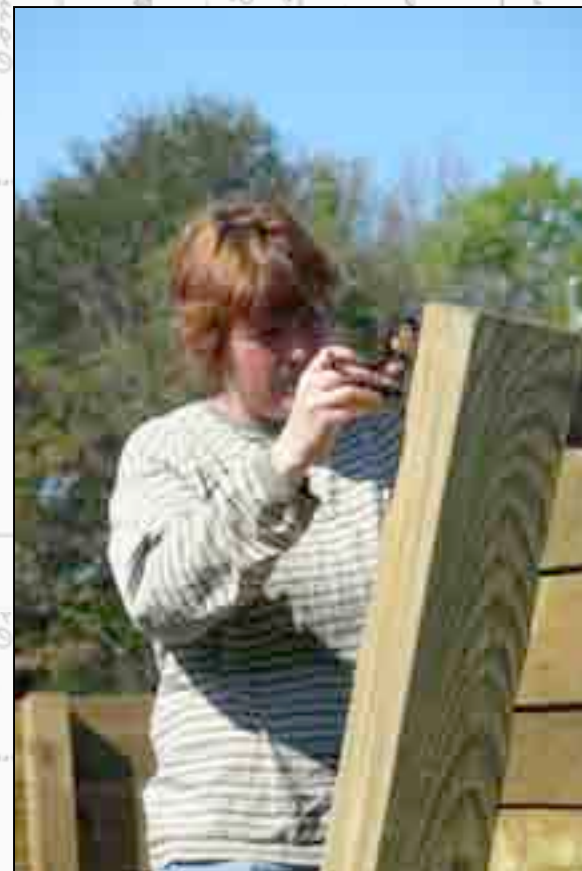
Amy prepares to cut the top portion of the post to make it even with the ground
