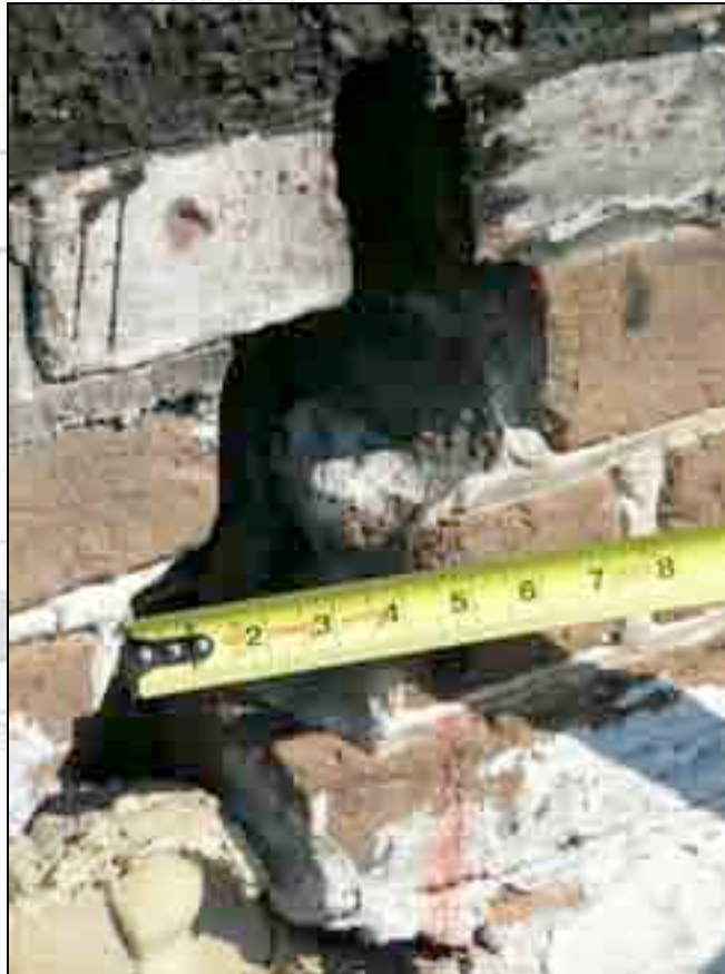
One point in the crack is measured at four inches.
