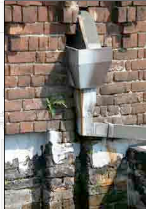
A faulty gutter system contributes to the mortar deterioration and wood rot along the edges of the Boiler House and Compressor Room.
