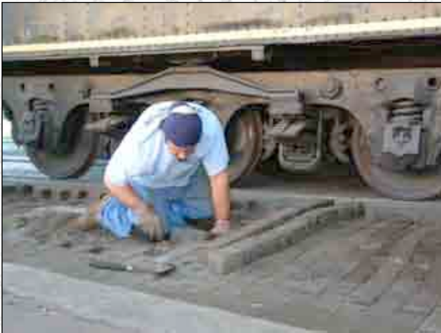
Bill Hersch removes the original woodblocks to prepare the area for testing.
