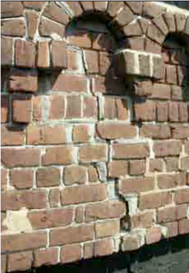
A large crack has formed in the eastern wall of the Boiler House.
