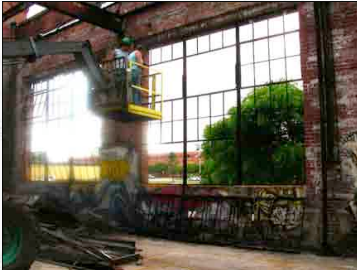
Amy Grace and Jeremy Bloomfield remove the steel window frames to start the next phase of window restoration at the Coach and Paint Shops.
