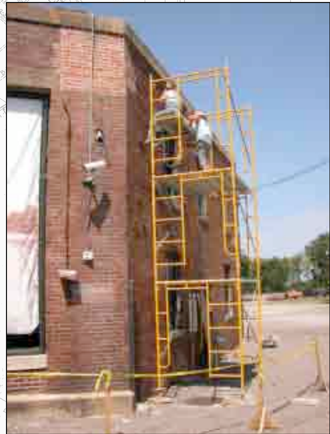
Using tungsten-tipped chisels, Brandi Hayes, Katie Purcell and Megan Kelly repair cracks in the mortar joints.
