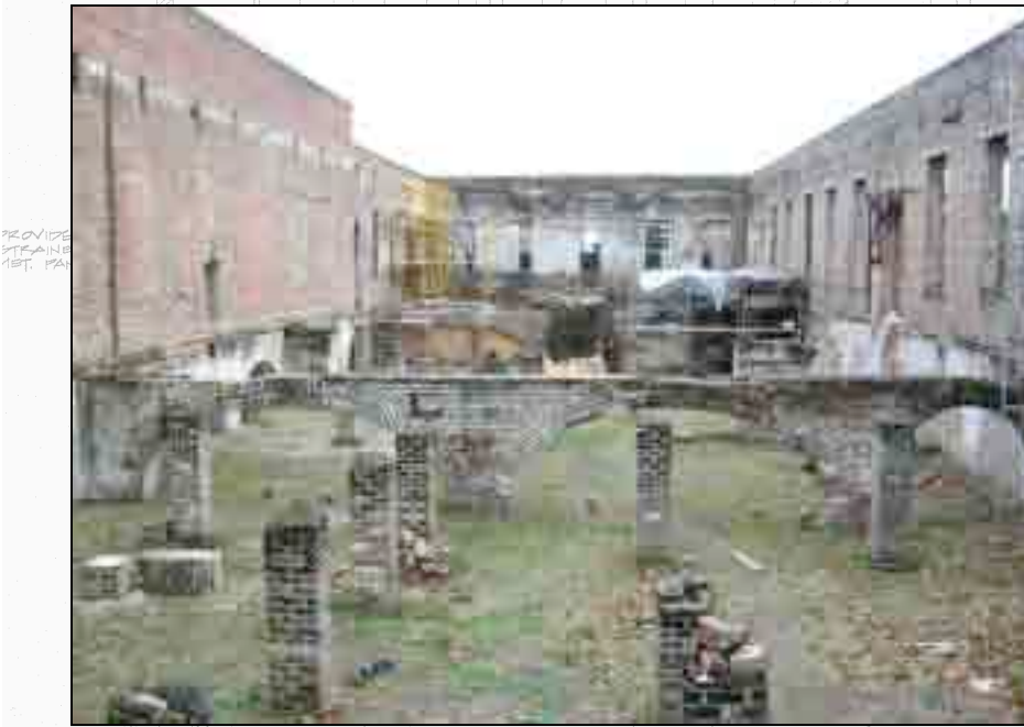
View of foundation arches shortly after masonry restoration began. Most areas were severely deteriorated and unstable.
