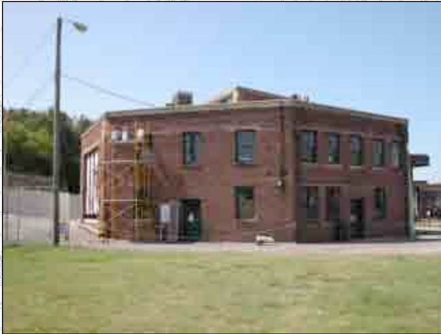
Scaffolding was set up for masonry repairs outside the main entrance of the gift shop.
