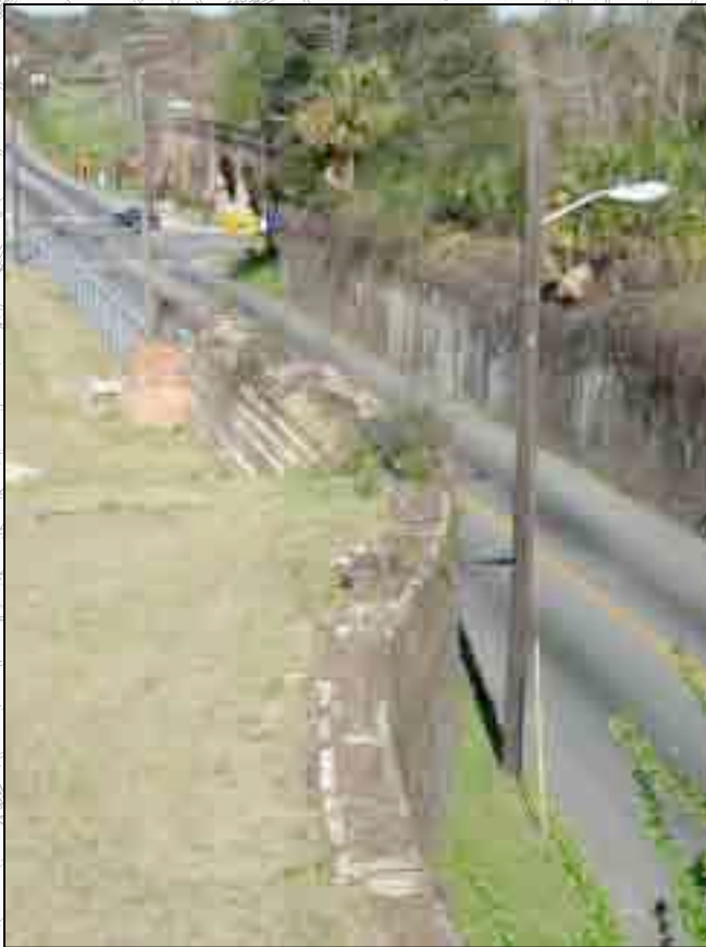
Aerial view of retaining wall overgrown with vegetation.
