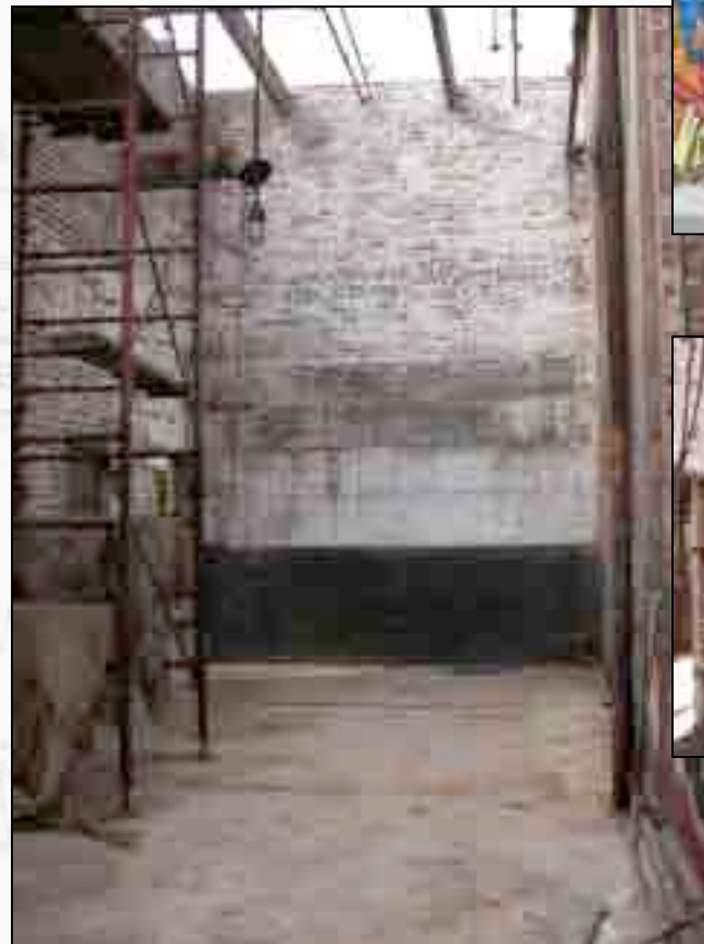
A good example of the building's original paint color scheme of bottle green at the four-foot wainscot and white above was revealed after the shelves were removed.
