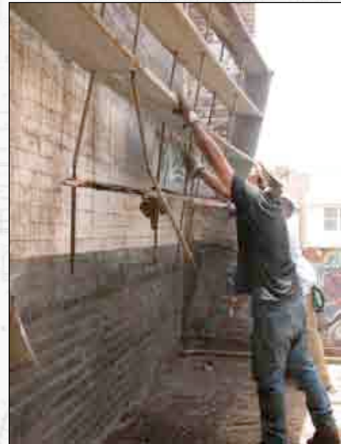
After loosening the screws, Kevin and John take the remaining structure down.
