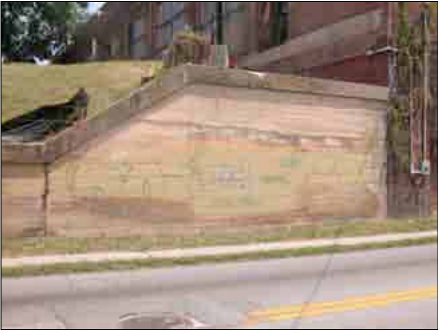
Before graffiti was removed.
