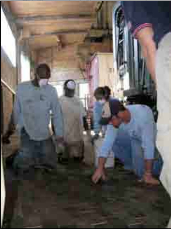
Alongside his crew, Project Engineer Bill Hersch lays the last wood block.
