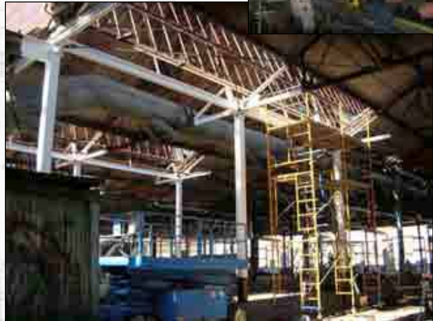
Scaffolding has been set up to repair the first of five valleys of the prototype area.
