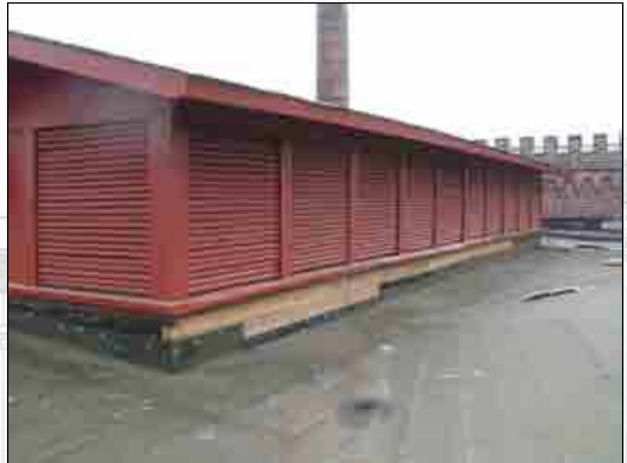
An historic paint analysis was performed to determine the original paint color.
