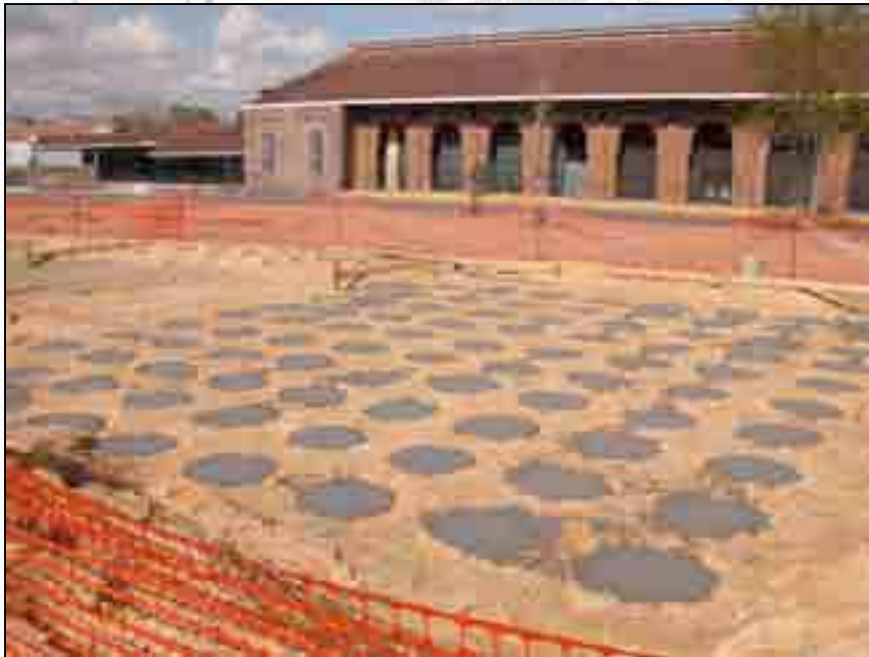
View of memorial walk shortly after construction began. Concrete piers were poured.
