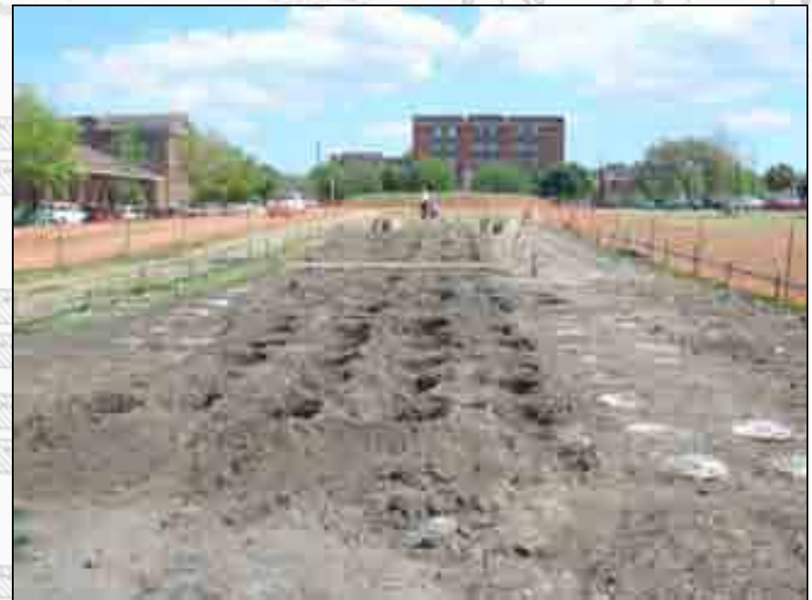
Concrete piers were poured into the ground in preparation for the granite markers.
