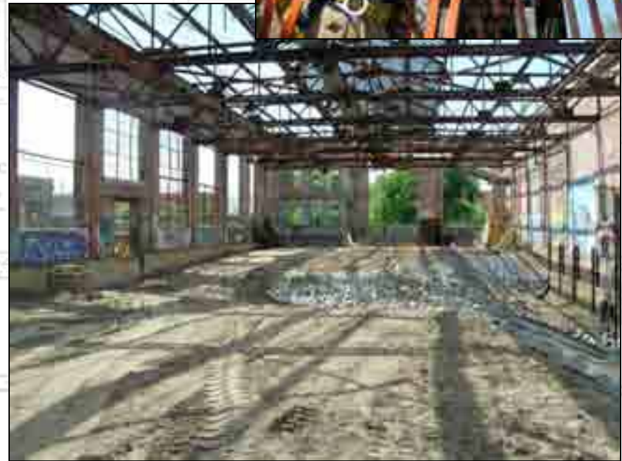
Current view of Coach Shop. Sashes have been removed from 8 ½ window openings to date (3 of the window openings are not in this view).
