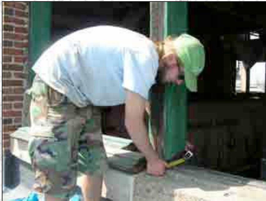
Nathan Harris measures a deteriorated segment that needs repairing.
