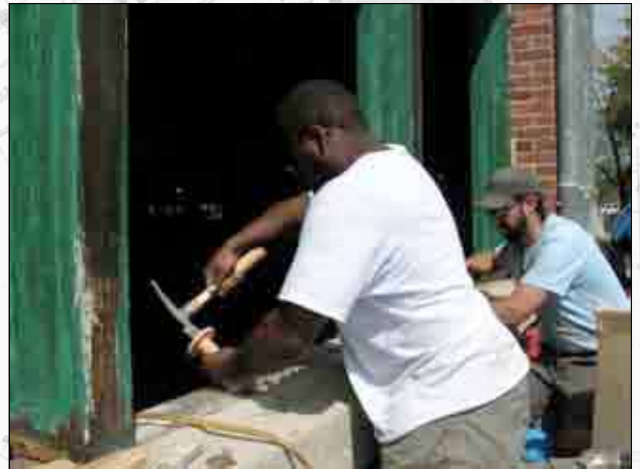
Allan Ballard and Justin Wiedenbach prepare the concrete sill for the window frame.
