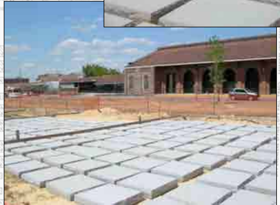
Current view of memorial walk with newly laid granite markers placed on top of the concrete piers.
