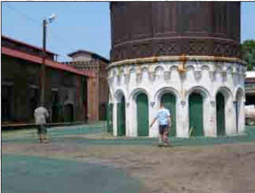
Chris Fisher and Ryan Griffiths install barriers to keep people from walking on the newly seeded grass.
