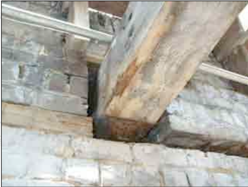
View of rafter suffering from water and termite damage before repairs were done.
