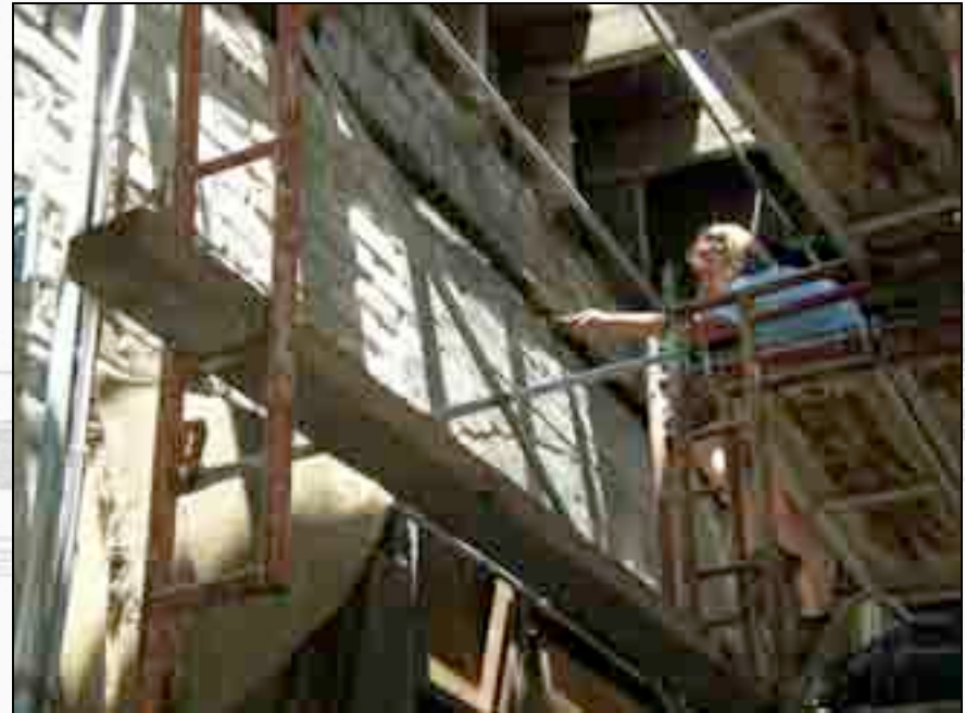
After digging out deteriorated mortar from the wall, Lissa Schwab rinses it away before repointing.
