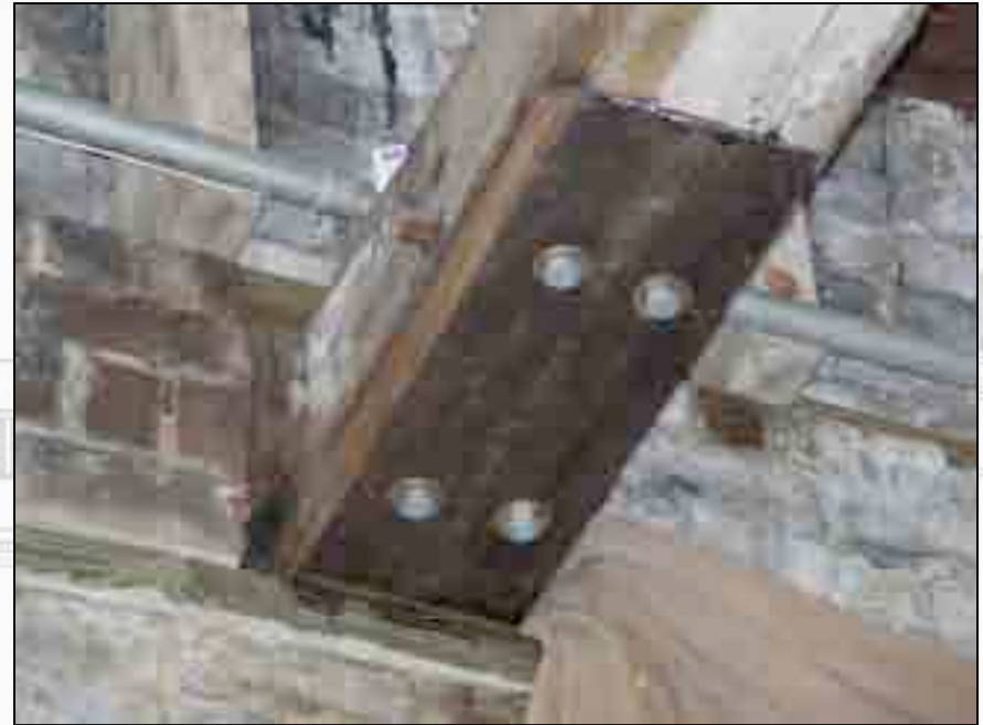
View of historic rafter with new sill and modified Dutchman repair. Masonry surrounding the rafter was also repaired.
