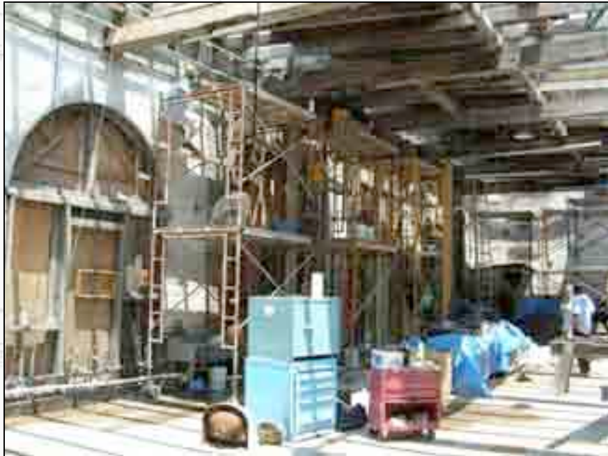
The CHS Preservation Team is currently repointing the north wall of the Compressor Room.
