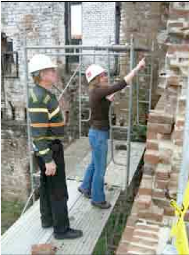
Becki points out areas of structural concern to Hunter.
