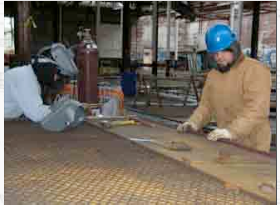
Chip DeYoung (right) lines up insertion holes on the original deteriorated steel frame of the window guard in order to fabricate a new one.
