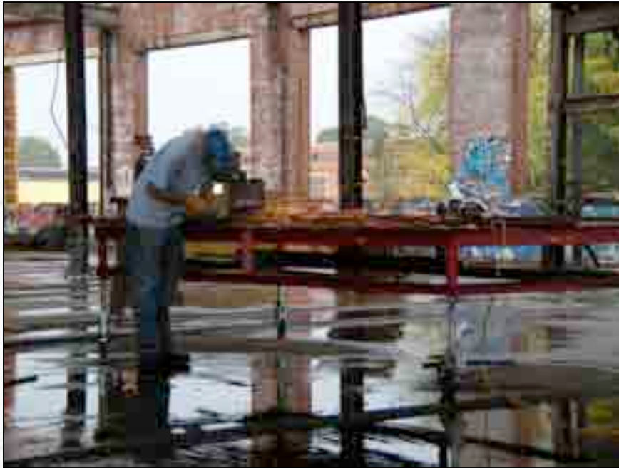
Joe Rothwell heats the wire ends in order to straighten and remove them from the steel channel frame.
