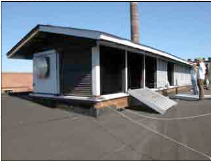
Nathan Harris and Amanda Smaridge help Kurt Benton (inside monitor) reinstall restored louvers into the monitor.
