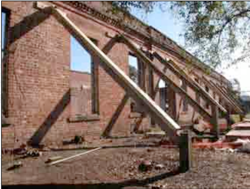
Older bracing on the wall was recently reinforced or replaced.
