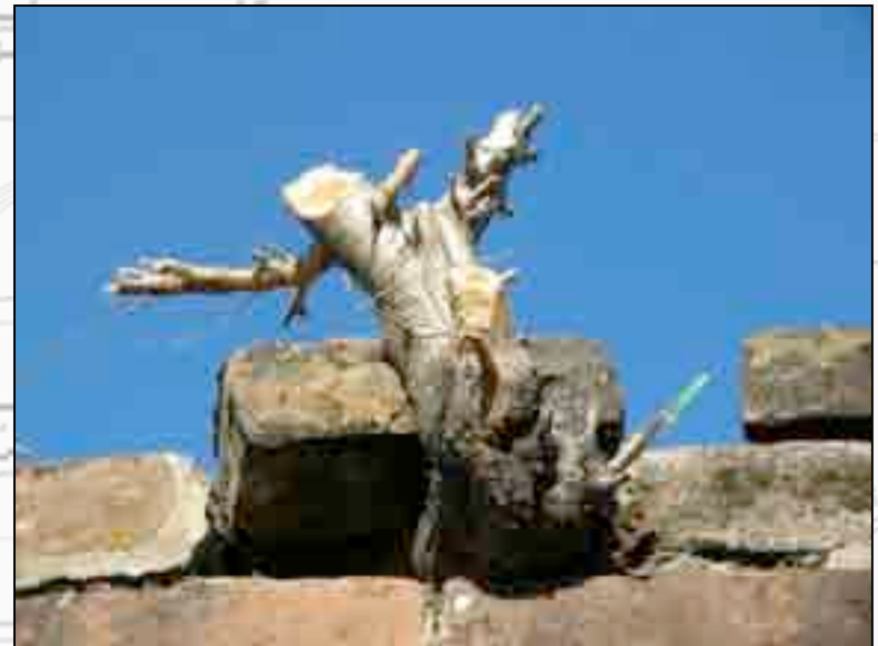
View from Louisville Road. Root can be seen dislodging the brick from the rest of the wall. In order to remedy this problem, the team drilled holes into the remaining trunk and root system and applied a tough brush killer.
