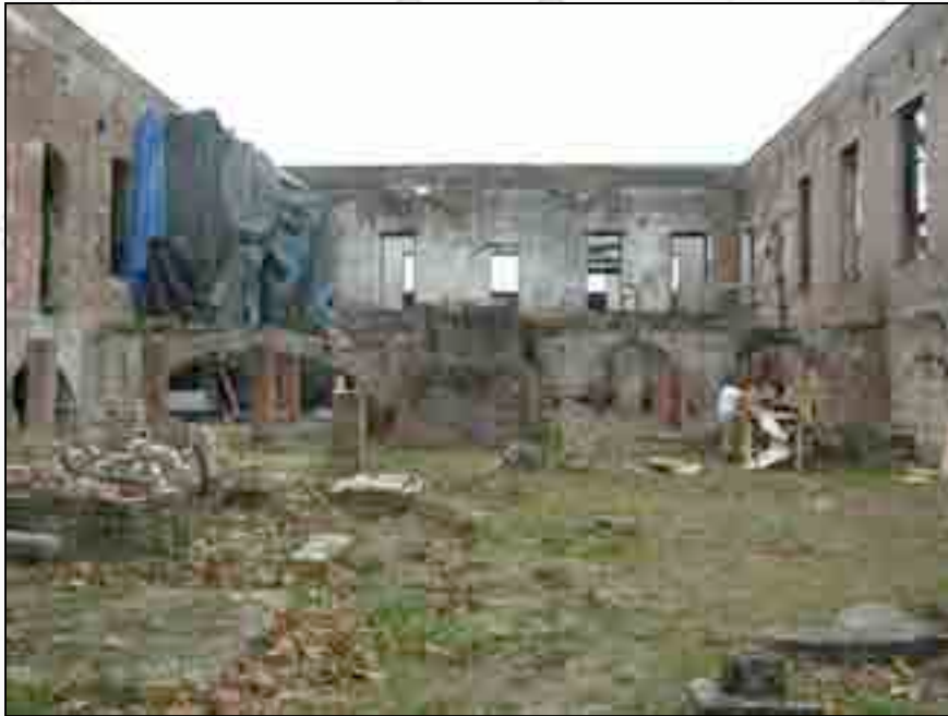
View of Carpentery Shop shortly after Southern Preservation Systems began reinforcing the foundation arches for repairs.
