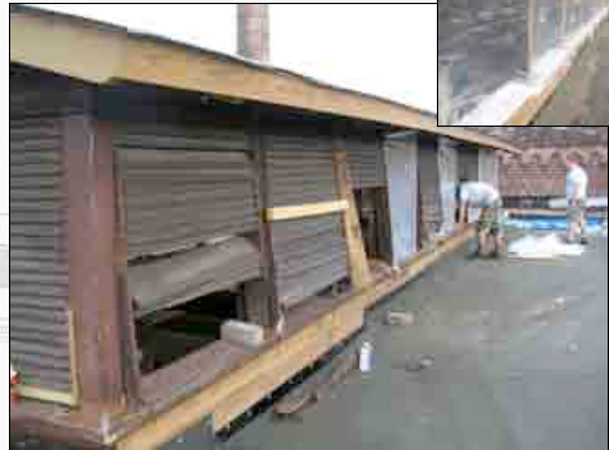
To keep rain from entering the Compressor Room, Preservation Team members Nathan Harris and Ryan Griffiths covered the openings with a protective plastic sheathing.
