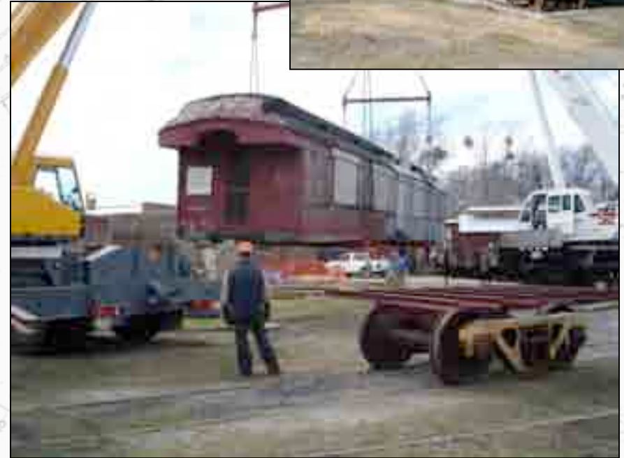
Augusta car in mid air as it was being transferred onto railcar trucks.
