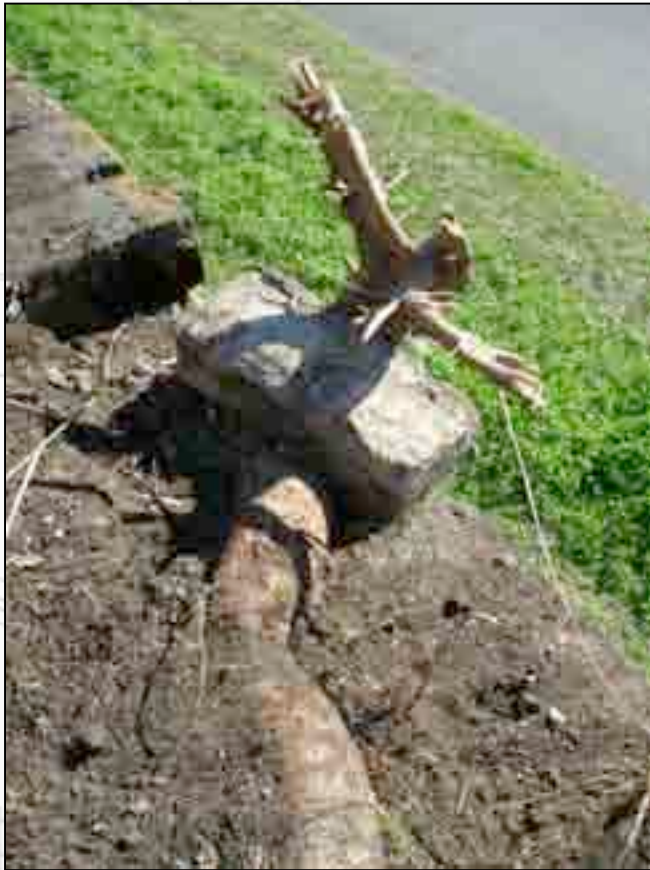
View of brick from top of masonry wall. The root can be seen growing through the wall.
