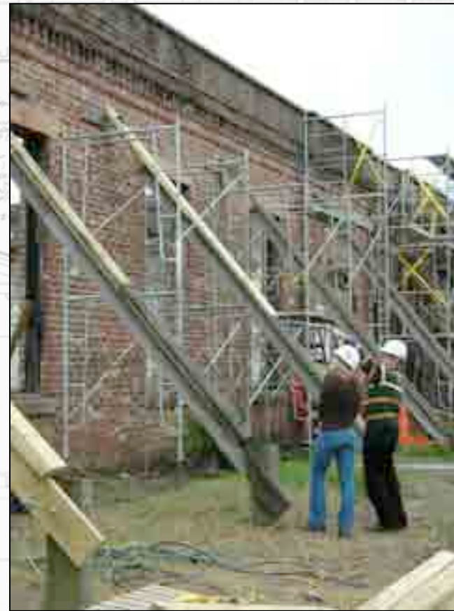
Hunter and Becki discuss the current bracing on the west wall of the building.
