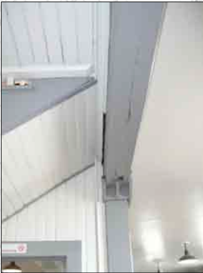
View of beam before repairs.
