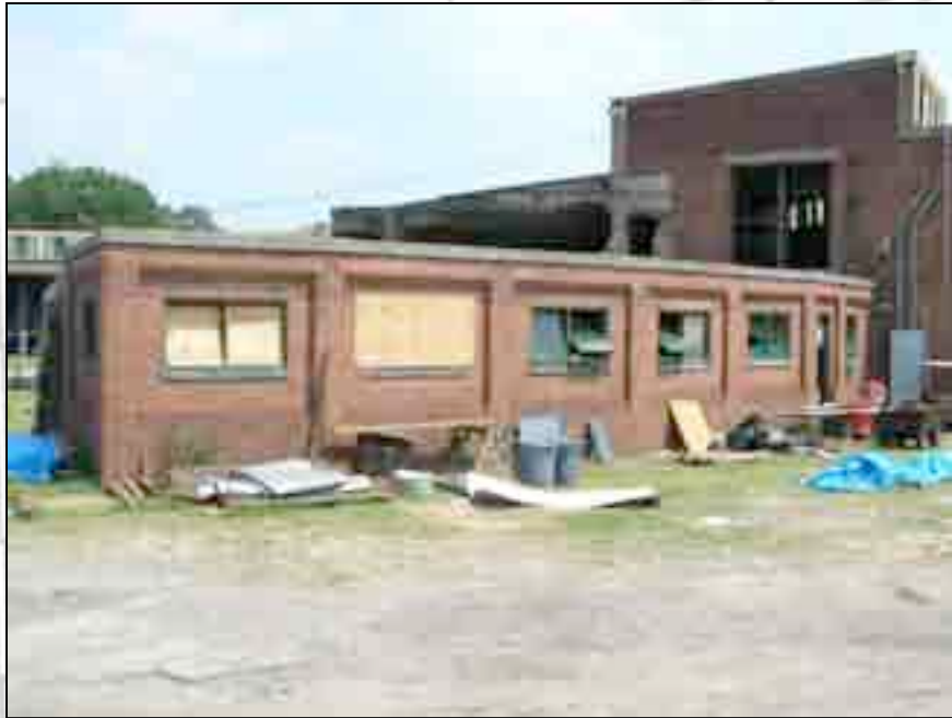
Colored Washroom shortly after window restoration project began. In this photo, only two sets of windows have been removed for repairs.
