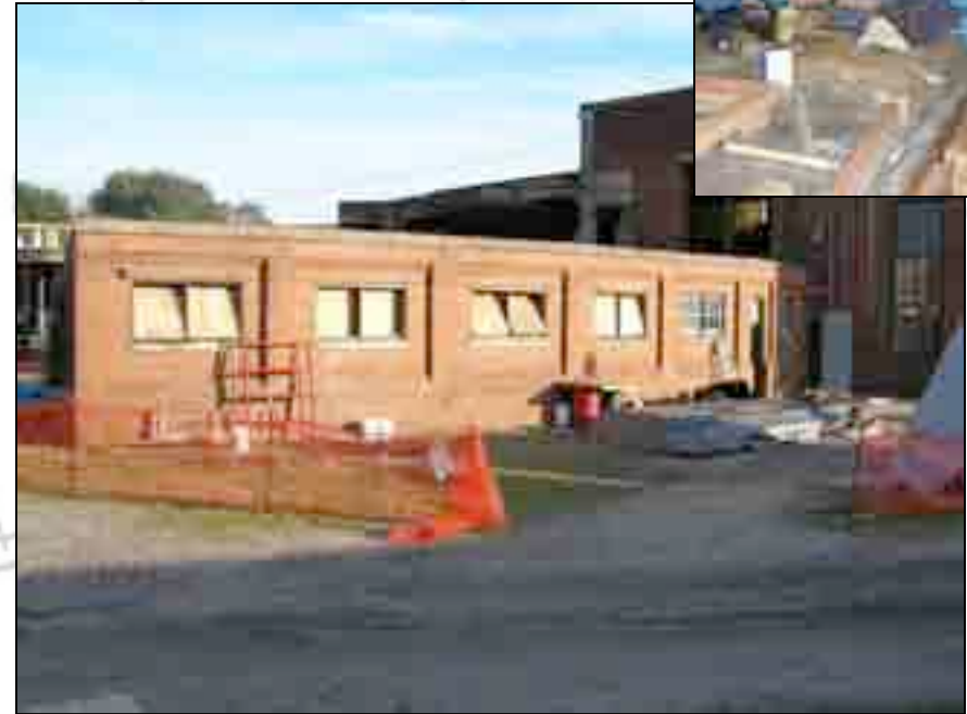
Current view of the Colored Washroom. Two windows have been reinstated on the right.
