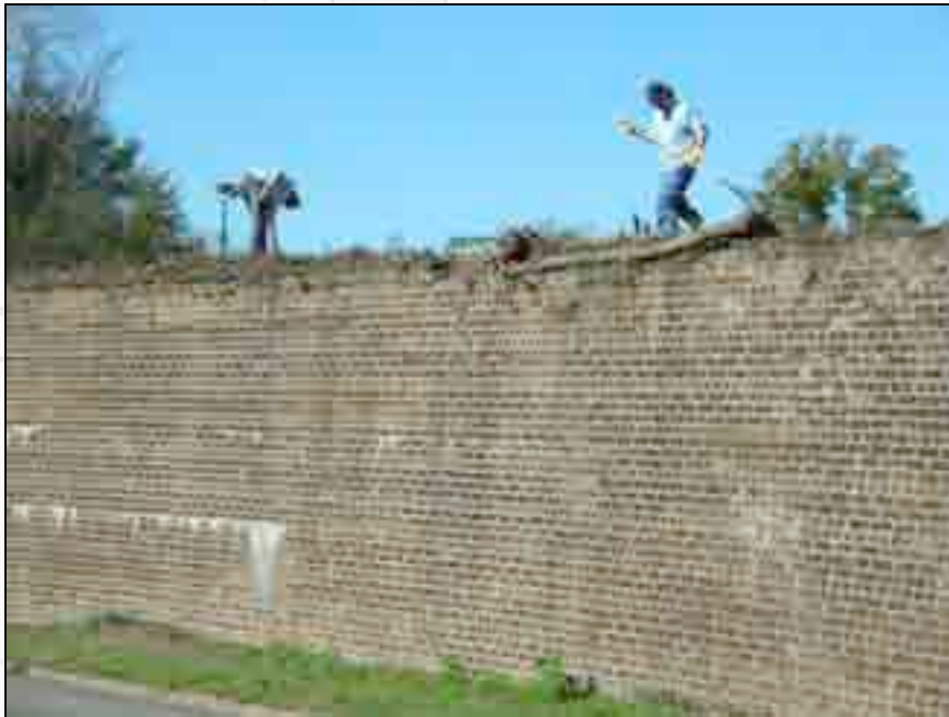
John Passmore and Kevin MacMillan clear brush from the masonry retaining wall along Louisville Road.
