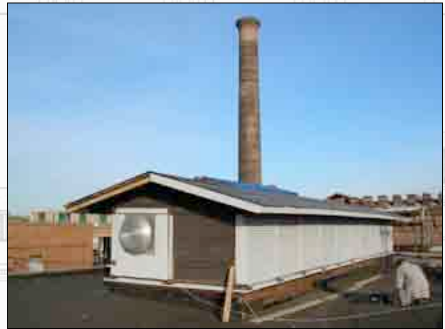
Current view. All of the louvers on the monitor have been restored and reinstalled.
