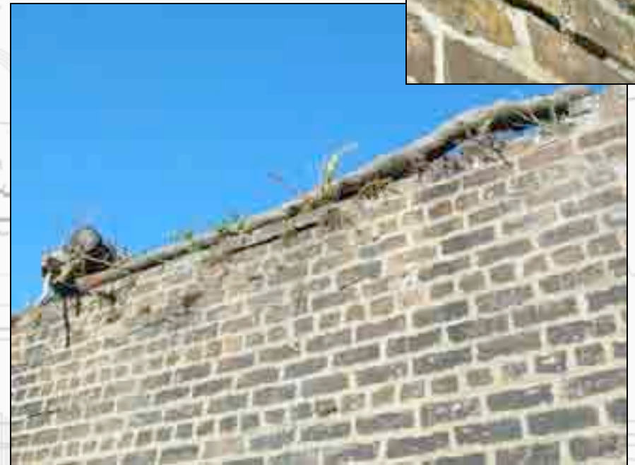
View of tree and its roots growing along the masonry retaining wall.
