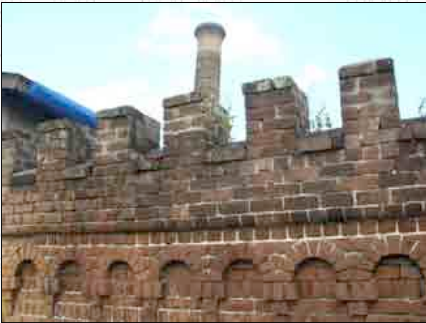
Close-up view of deteriorated mortar joints
