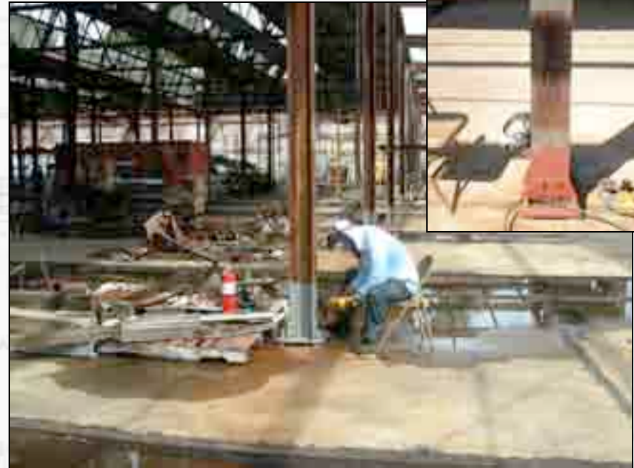
Joe Rothwell grinds a column to help conceal most of the weld seam. A small portion of the interior seam will be left visible to distinguish from the original and repaired parts of the column, a standard practice in historic preservation.
