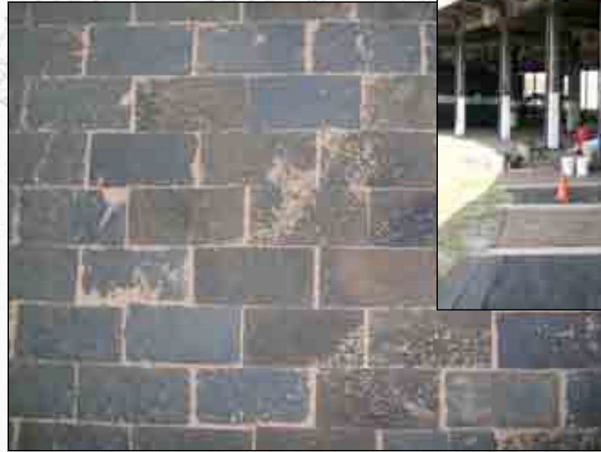
View of restored woodblock floor before a sealant is applied. Original woodblocks were used when possible.
