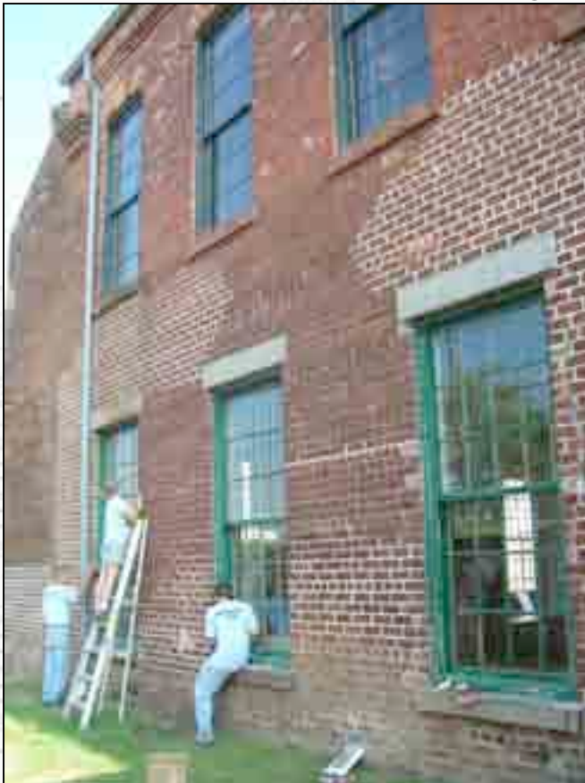
Charles, Amy, and Eric scrape and sand the window frames before repainting.
