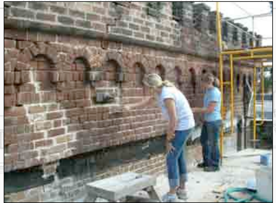
Newcomers, Brittany Barton and Tarin Erickson, take out deteriorating mortar from masonry joints.
