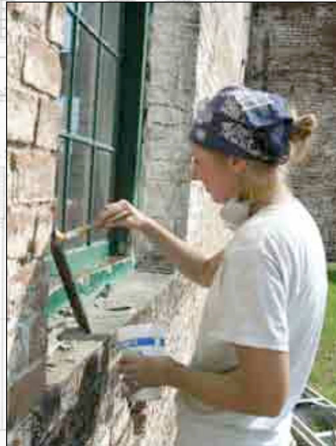
Amy applies Boracare to a Dutchman repair on the window frame. The application prevents termites and biological growth from damaging the wood.
