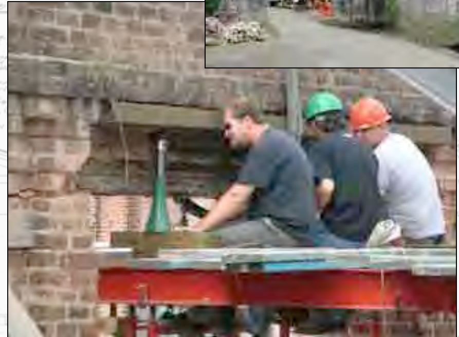
Justin Rowles, Bryan Law, and Project Manager Terry Koller (l-r) use a screw jack to hold the temporary lintel firm while they secure it in place.
