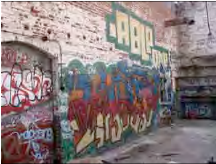
East wall of the Paint Storage Room located on the main floor before graffiti was removed.
