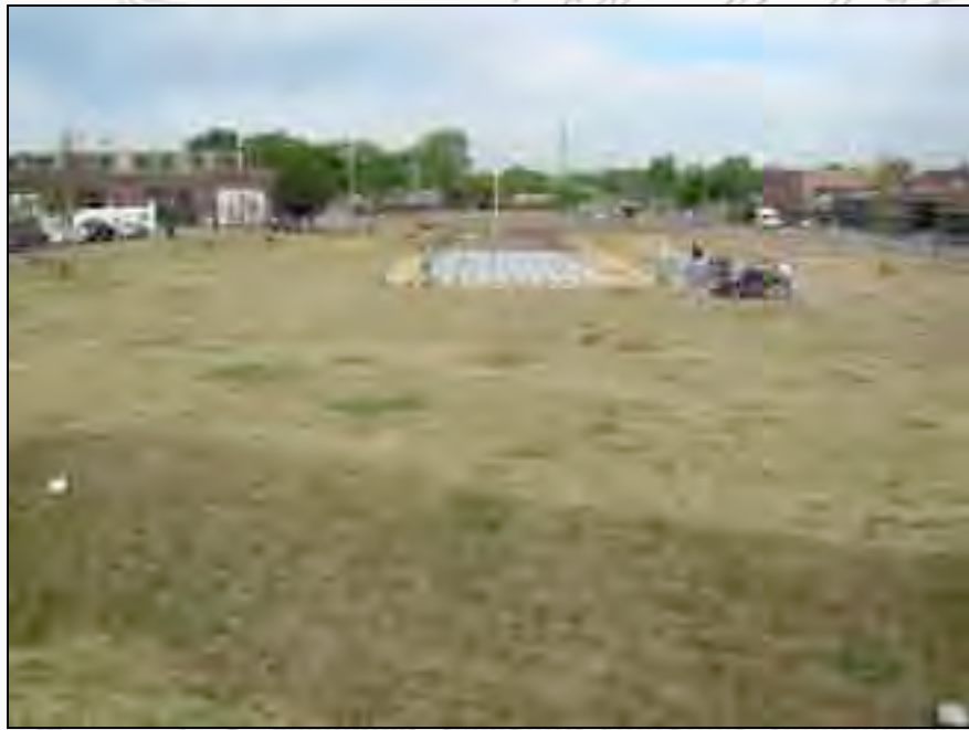
Preservation Team members place the remaining stones in the memorial walk and finish preliminary grading.
