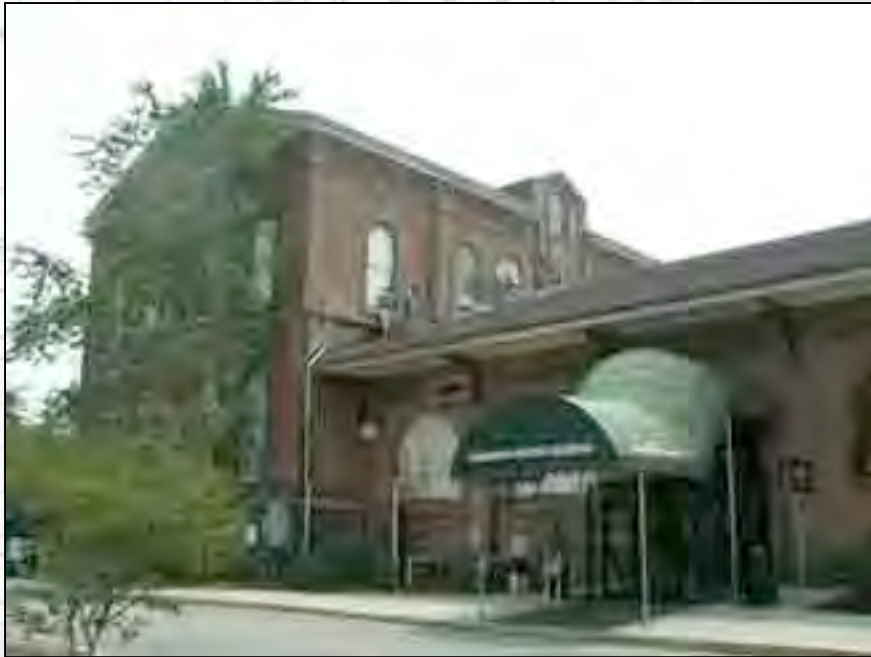
Exterior view of CHS offices and Savannah History Museum. Preservation Team members remove deteriorated mortar while Project Manager Eric Davenport assesses the windows.
