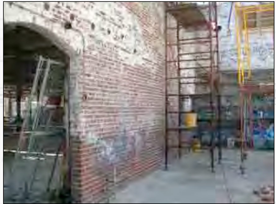
Current view after graffiti was removed.
