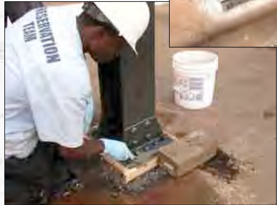
Using a wood form, James Jackson grouts the space between the column and floor with concrete.
