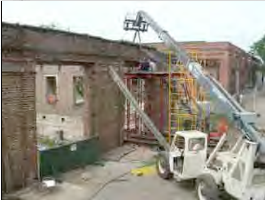
A forklift keeps the wall secure while the steel crew works on the lintel.
