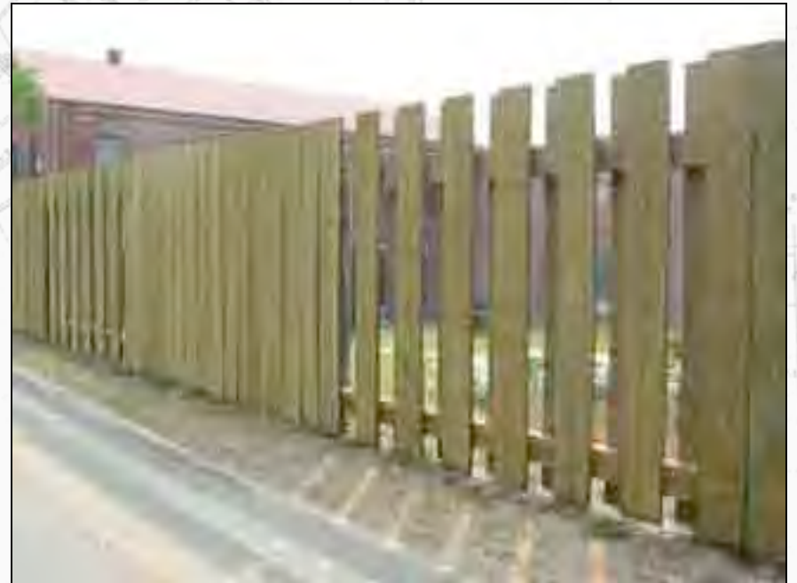
View from Purse Street. Two sections of the fence were designed so that the garden could still be seen from the street.
