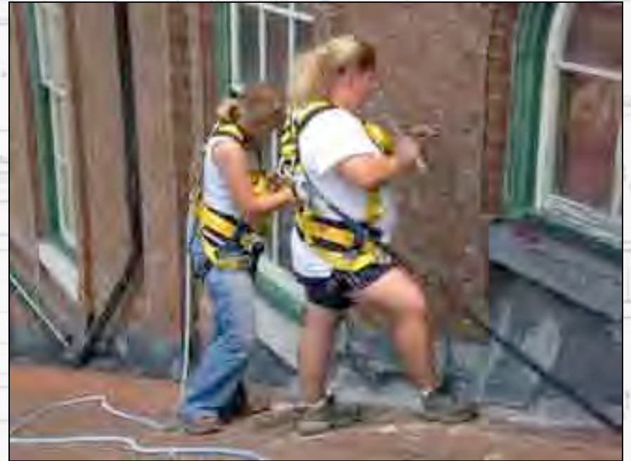
Attached to harnesses on top of the roof, Preservation Team members Tarin Erickson and Candice Leite investigate the condition of the mortar from the second story west façade of the Visitors Center.
